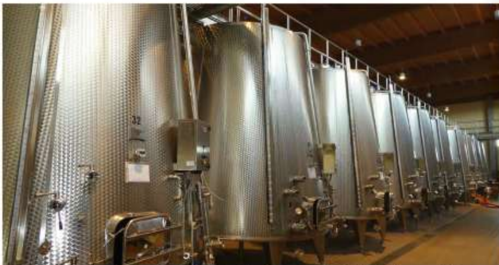
Stainless steel fermentation tanks at Donnafugata's Vittoria winery. They do not use any oak on this site as the wines are quite delicate
